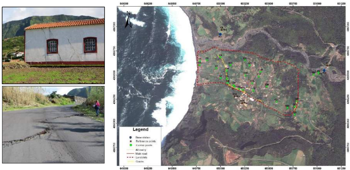
Figure 3. On the left, pathologies verified in housing and streets. On the right, delimitation of the unstable mass of the Fajãzinha and spatial location of the topographic network.
