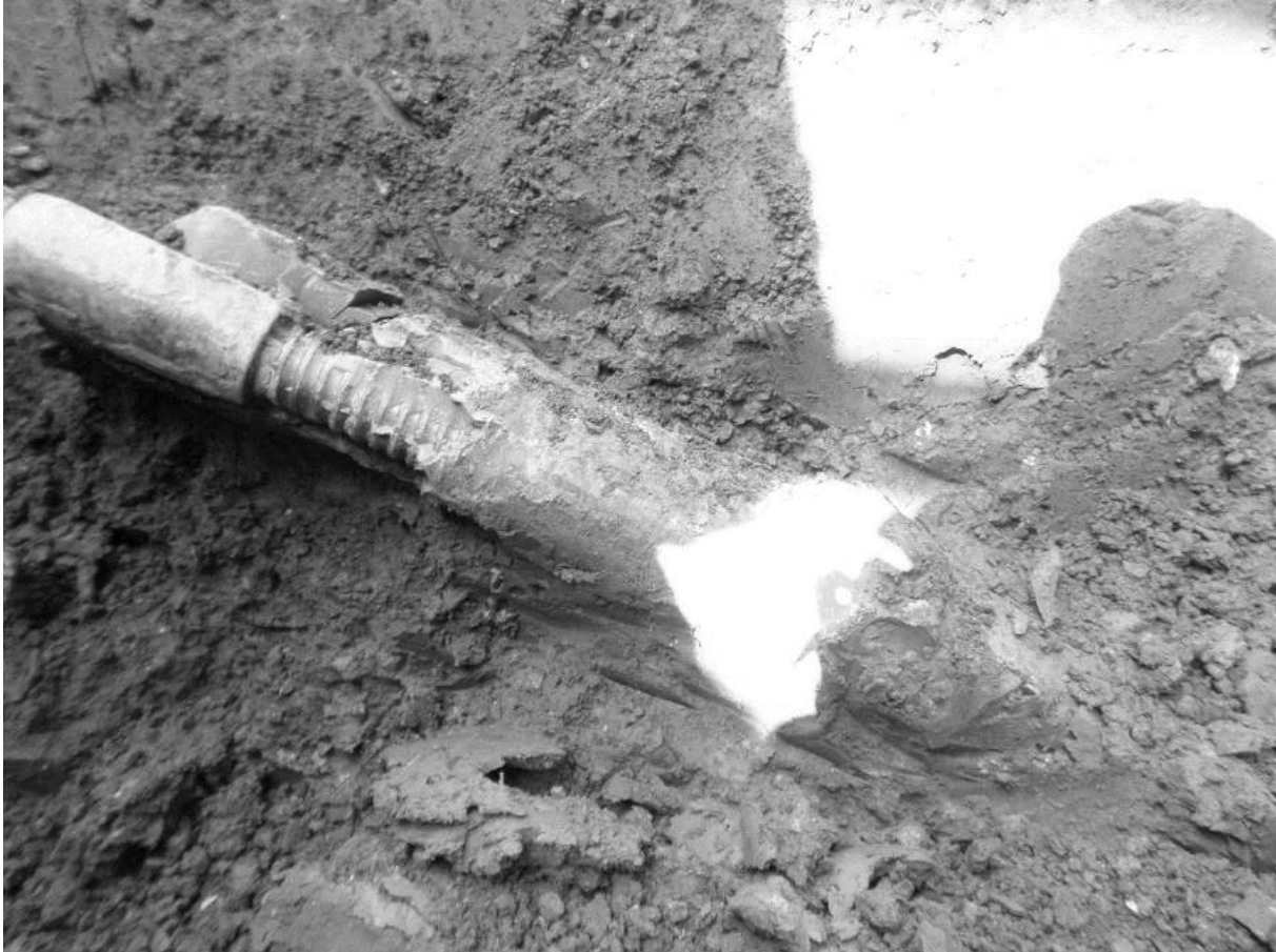
Figure 5. Poor grout of the injection bore anchor
