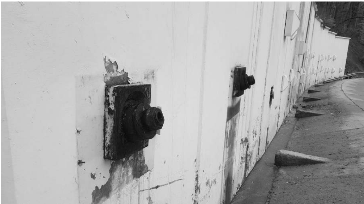
Figure 4. Corrosion of the construction
